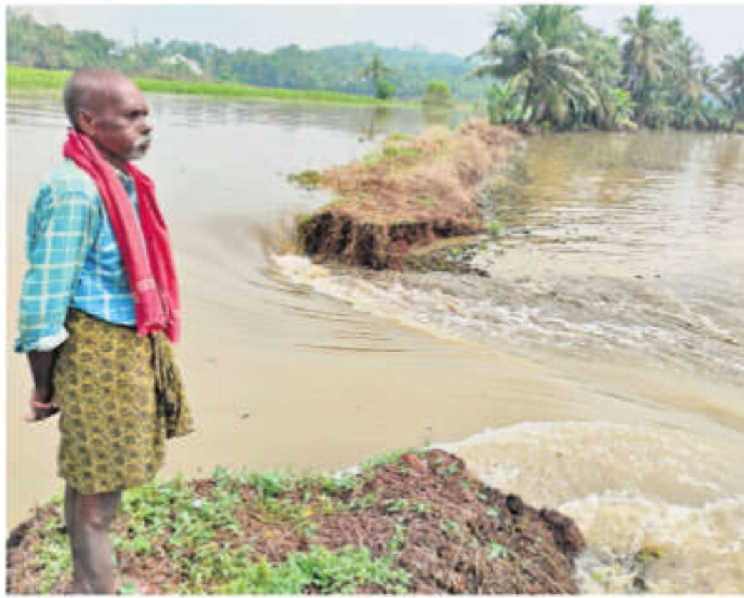
The bund breach at the Vadakkumpuram paddy polders, at Kollad near Kottayam, caused by heavy rain has damaged the newly sprouted plants in the area | EXPRESS
