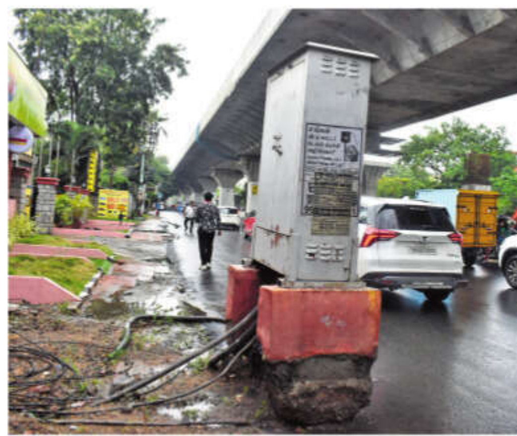
A pillar box of Tangedco uprooted and kept aside on Avinashi main road near 'The Grand Regent Hotel' posing threat to motorists | S SENBAGAPANDIYAN
