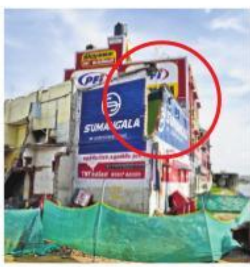
Chennai Metro Rail has agreed to undertake the repair work on the portion of the building that was damaged | MARTIN LOUIS
