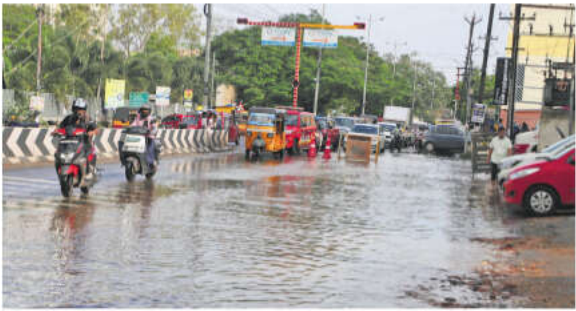
Motorists wade through rainwater accumulated on a damaged stretch of road at Lakshmi Mills in Coimbatore on Friday following a spell of rain | s SENBAGAPANDIYAN
