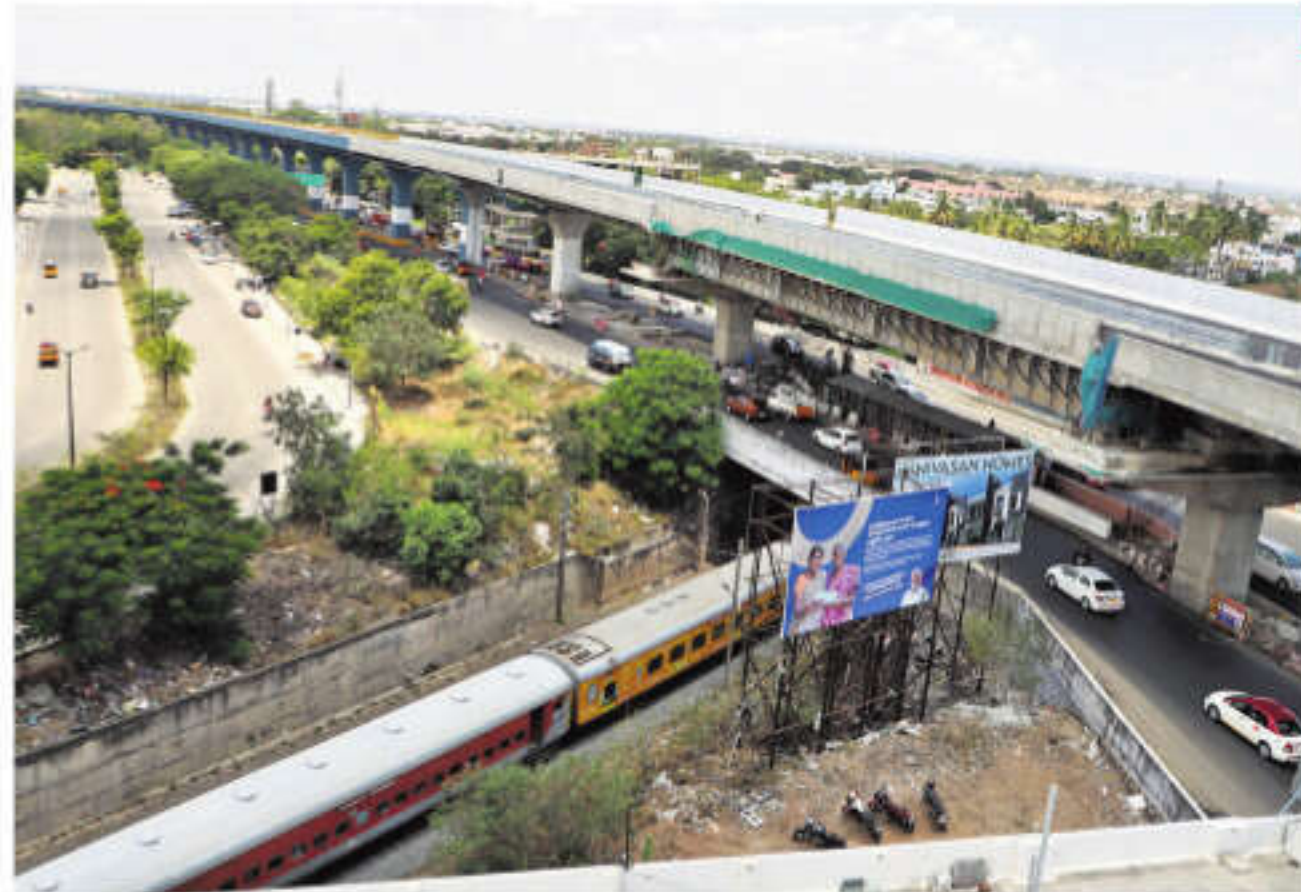
Special Projects Wing officials confirmed that the crucial deck works near the Hopes junction, carried out above live railway tracks and high-tension electric lines, have been completed | S SENBAGAPANDIYAN
