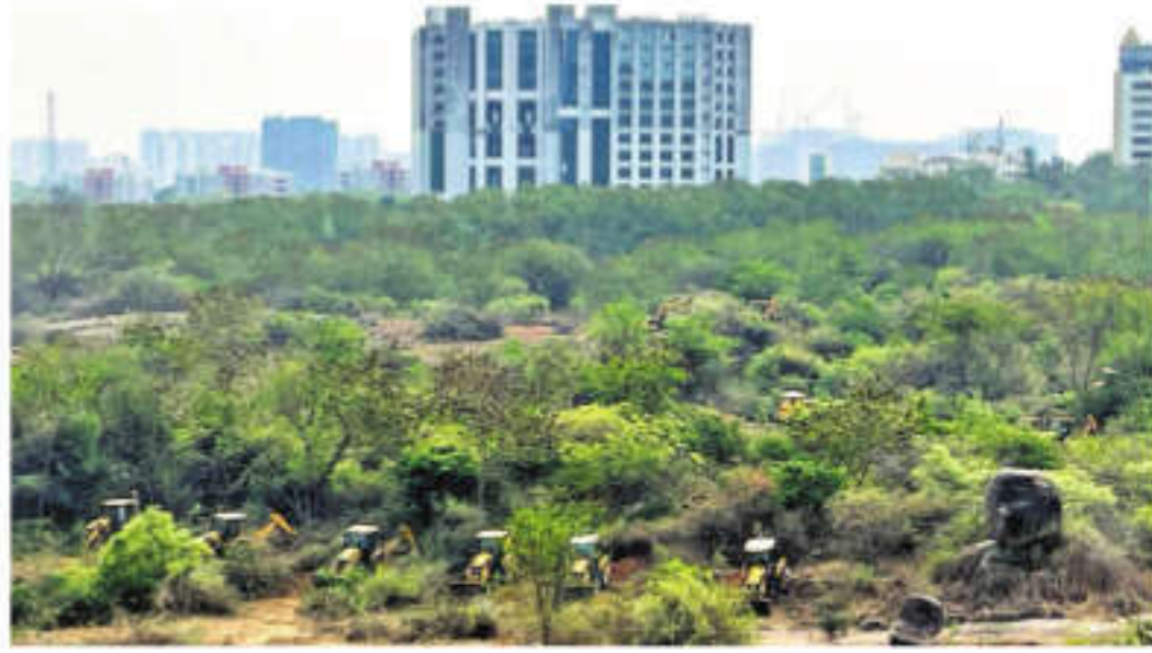
Excavators levelling land inside the University of Hyderabad campus in Kancha Gachibowli | EXPRESS
