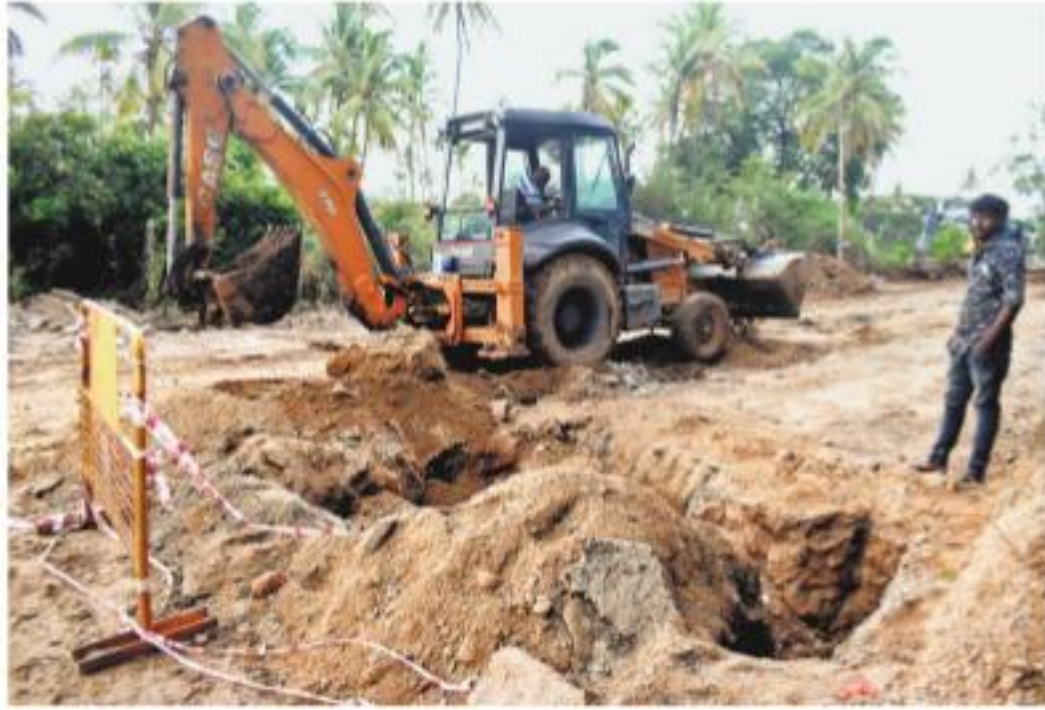
State highway department workers engaged in repair works after a portion of Puttuwaki road in Coimbatore caved in a few days ago | S SENAGAPANDIYAN
