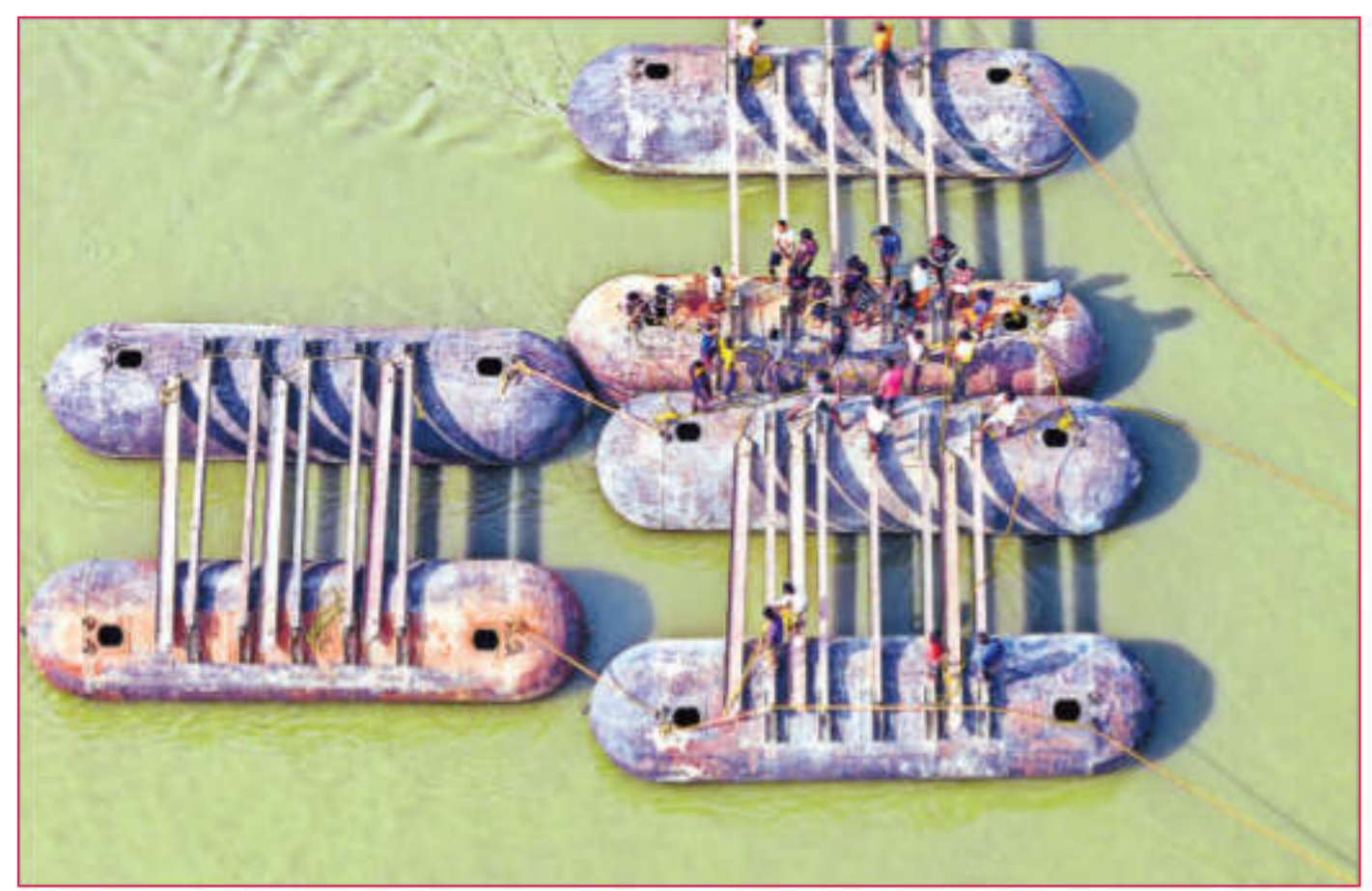
Labourers construct a pontoon bridge for the upcoming Magh Mela, in Prayagraj, on Sunday. The festival will take place from January 3 till February 15
