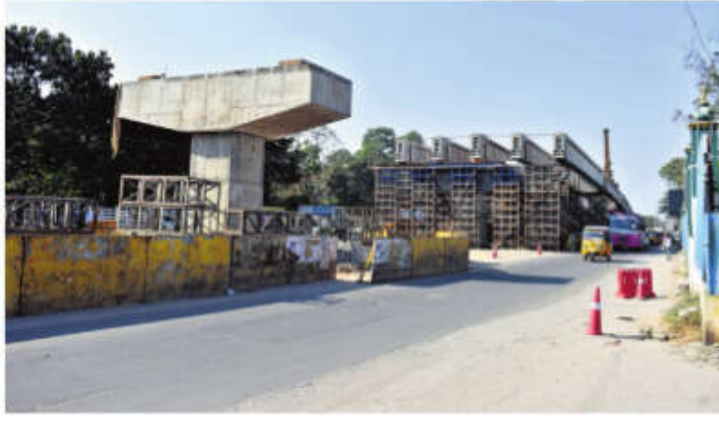
A flyover coming up at Saibaba Colony on Mettupalayam Road | S SENBAGAPANDIYAN
