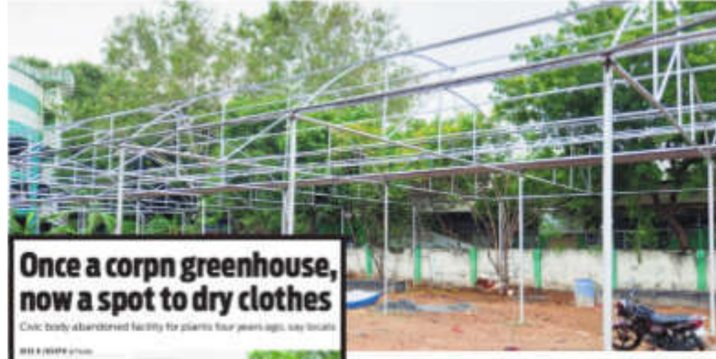
Once a corpn greenhouse, now a spot to dry clothes. Civic body abandoned facility for the plants four years ago, says locals
