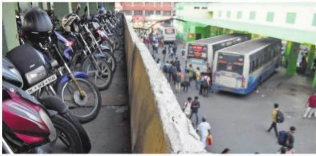
The dilapidated parapet wall in the parking facility of Gandhipuram central bus terminus in Coimbatore | S SENBAGAPANDIYAN
