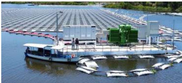
AMBER TO GREEN. NGEL plans to initiate the process for filing DRHP after June. A file picture of NTPC Kayamkulam floating solar power plant
