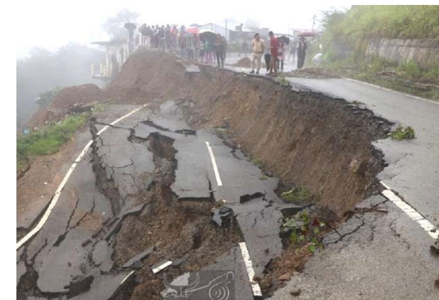
A portion of National Highway 702A collapses at New Colony in Zunheboto, due to the landslide, on Wednesday morning. - Photo: Correspondent
