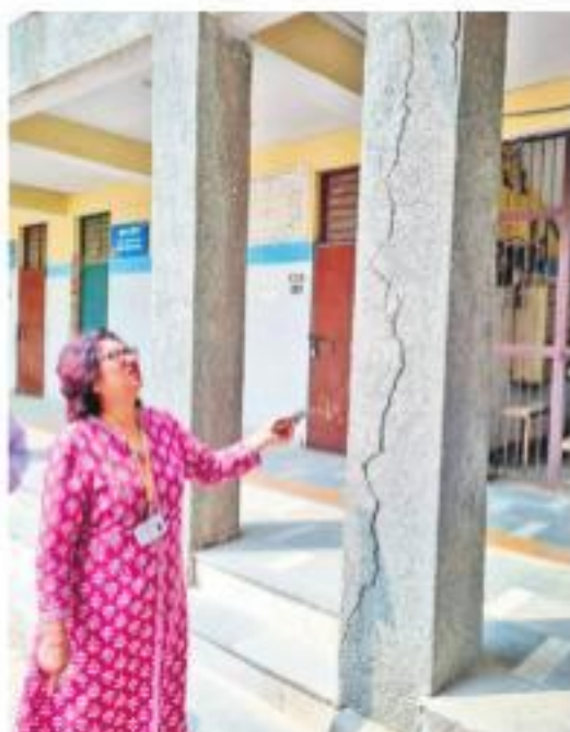
A DCPCR official checks a crack on a pillar at a school | EXPRESS
