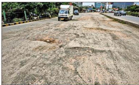
Trucks and dumpers frequently use the road to bypass the toll plaza, putting additional pressure on the weakened surface
