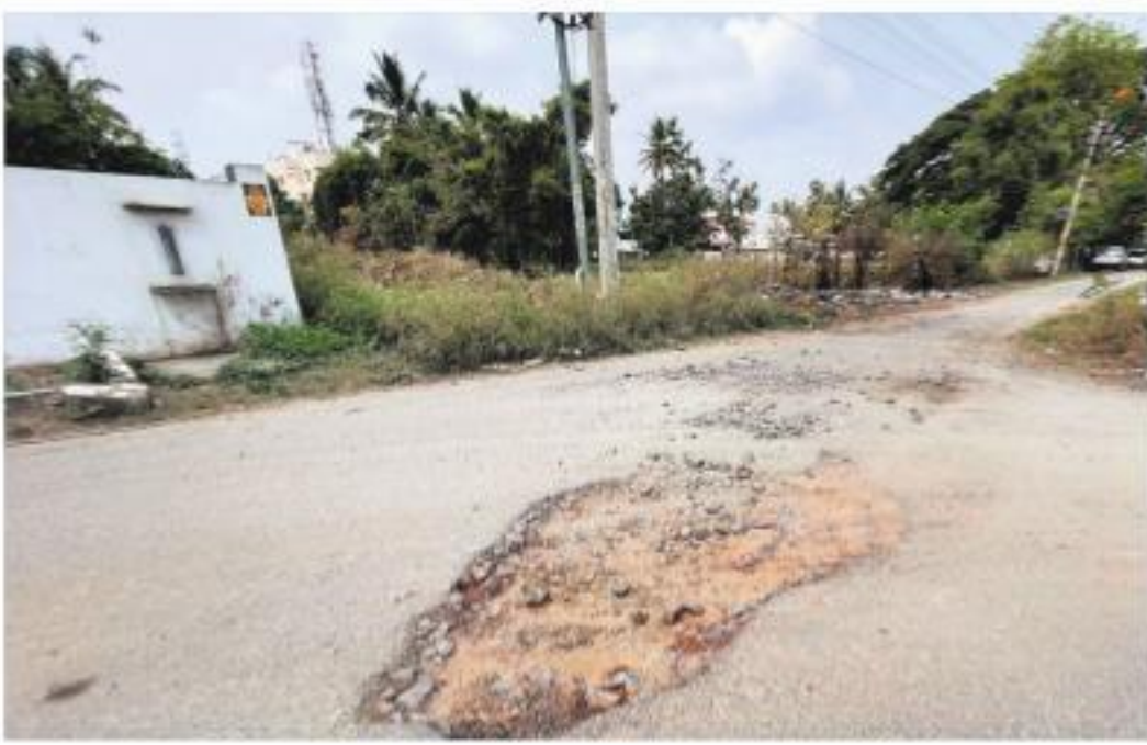
Roads near GN Mills flyover are damaged by movement of heavy vehicles | EXPRESS
